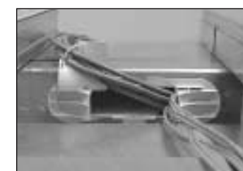
Bend Radius control for communication cables.
